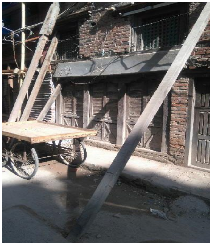
Fragilized buildings in Kathmandu.
