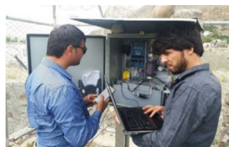
Configuration of system in Tangshiw village of Maimai district, Badakhshan province.
